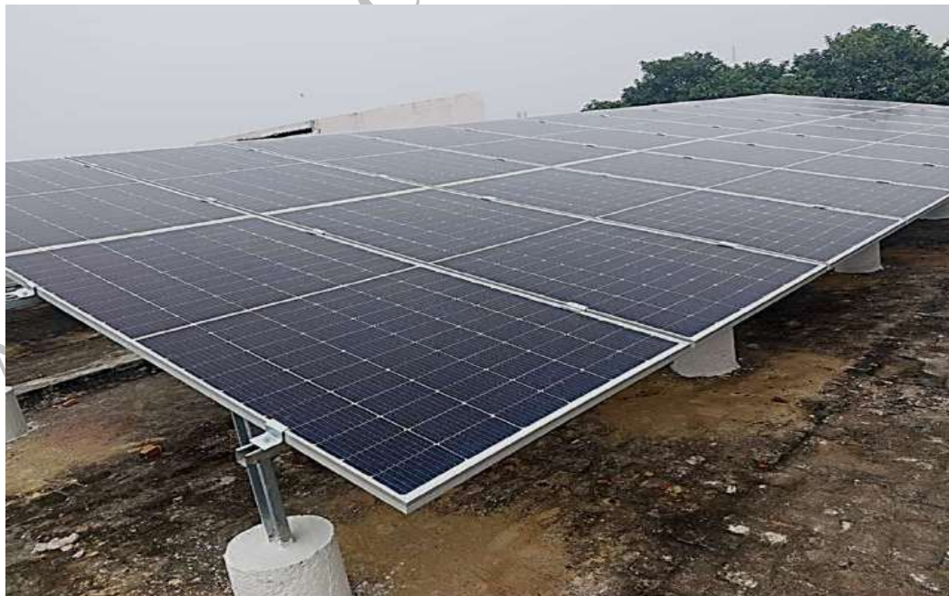
Solar Panels installed on roof top at Udai Pratap College, Varanasi, UP, India, to harness Solar Energy (Green Energy)
